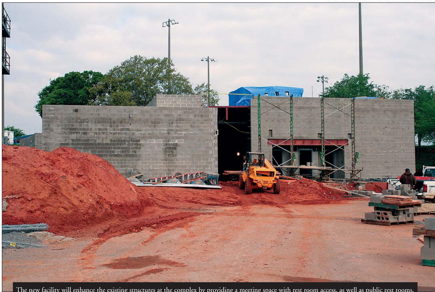
The new facility will enhance the existing structures at the complex by providing a meeting space with rest room access, as well as public rest rooms.
